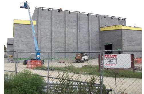
Work continues on the Danny and Willa Ellis Family Fine Arts Center on the campus of Fort Scott Community College.
